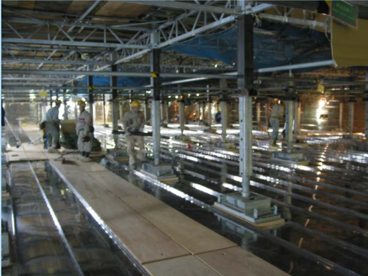
Special staging (12 levels) from bottom to top of a cargo tank for repairs (thousands of pieces of special stage materials similar to the staging in building construction)
