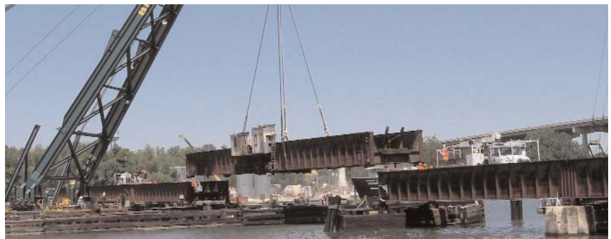
Following an emergency call Bisso Marine immediately mobilised the 600 tonnes capacity D/B Lili Bisso to Amelia, LA, to lift the Bayou Boeuf Railroad Bridge. The bridge had been struck by a tug and barge, resulting in significant damage. Upon arrival, Lili Bisso lifted the damaged 200 tonnes bridge span and placed it onto a deck barge. It was then transferred to a local repair facility. Upon completion of repairs, the D/B again lifted the repaired span and placed it back on to the deck barge. Subsequently, the span was put back on to its supports, allowing rail traffic to resume.
