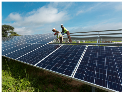
Senegal: Renewable Electricity from Solar Systems
