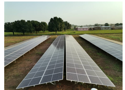
Mali: Rural Electrification
